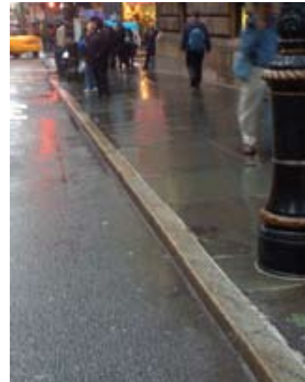
Saw-finish granite curb shown with historic bluestone sidewalk: Madison Avenue at East 51st Street, Manhattan
