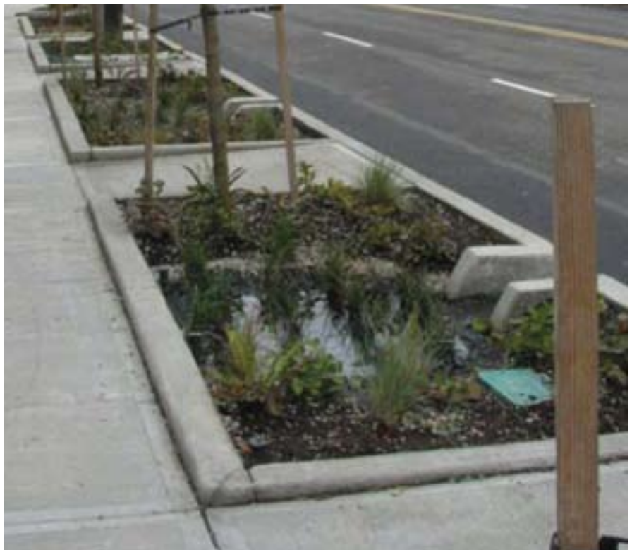
Stormwater–capturing tree pit with plantings: San Francisco (Credit: San Francisco Planning Department)
