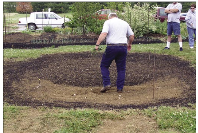
During this rain garden installation the area was over-excavated in sandy subsoil and backfilled with a soil amended with compost to increase organic matter content.
